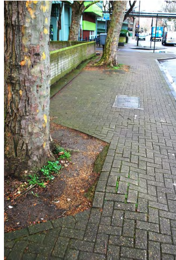
Image 3 – Stem bases of T108 & T107 – site supervision and hand working required to ensure surface roots are not damaged
